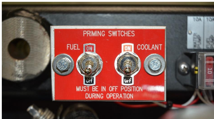
Figure 18 - Priming Switches Panel
