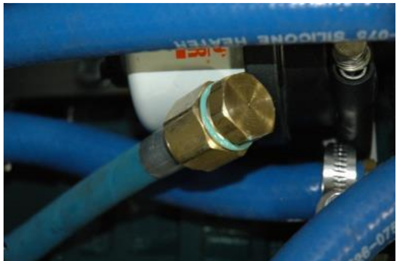
Figure 9 - Oil Pan Suction Hose
